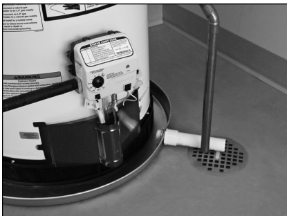
Figure 23 - Metal drain pan piped to drain.
