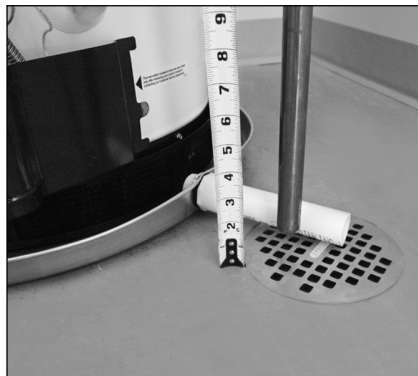
Figure 26 - Temperature and Pressure Relief Valve Pipe
