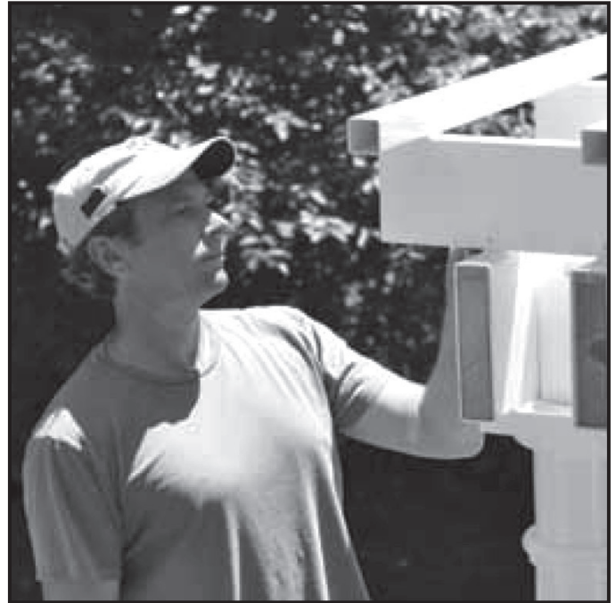
Prior to fastening the shades, sight the rafters and straighten shades as needed.
