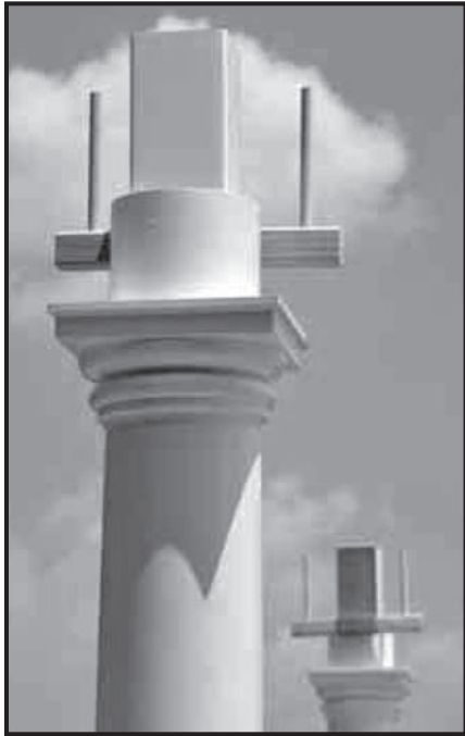
This is how the temporary beam holder should look when it is positioned to hold the beam during beam installation.
