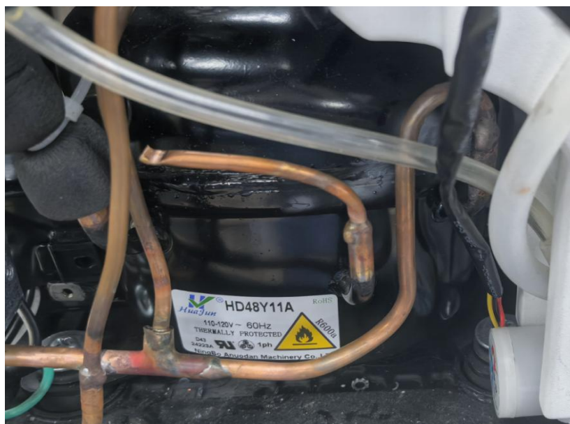
Photo 26 - Compressor HD48Y11A view
