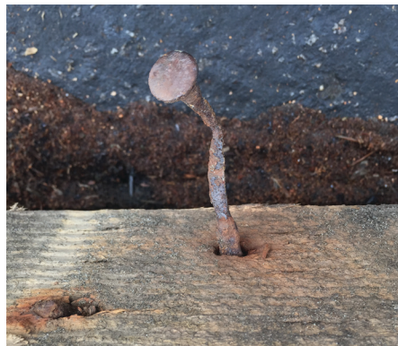
The effect of corrosion on HDG spikes.
