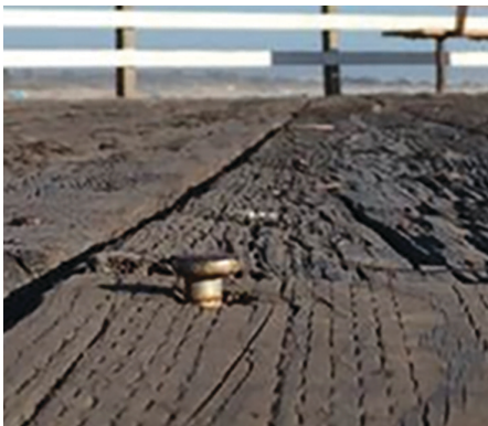
Spike pop-up hazard.
