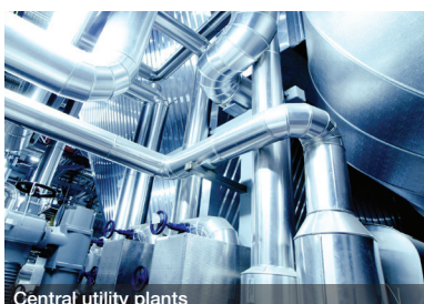
Central utility plants
