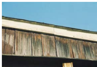
Not back primed. Weathered wood and mold
