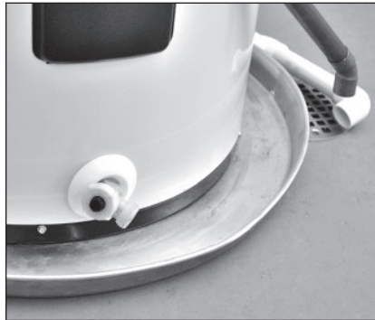
Figure 6 - A suitable drain pan piped to an adequate drain can help protect flooring from leaks and drips.
