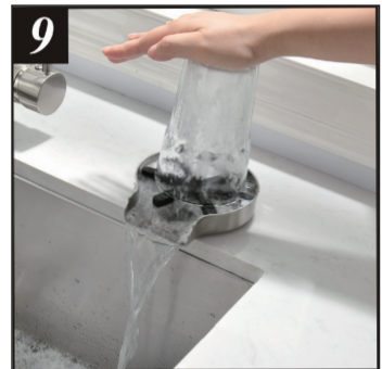
9 Turn on both water supplies at angle stops and check for leaks at all connections. Finish and enjoy your easy life.
